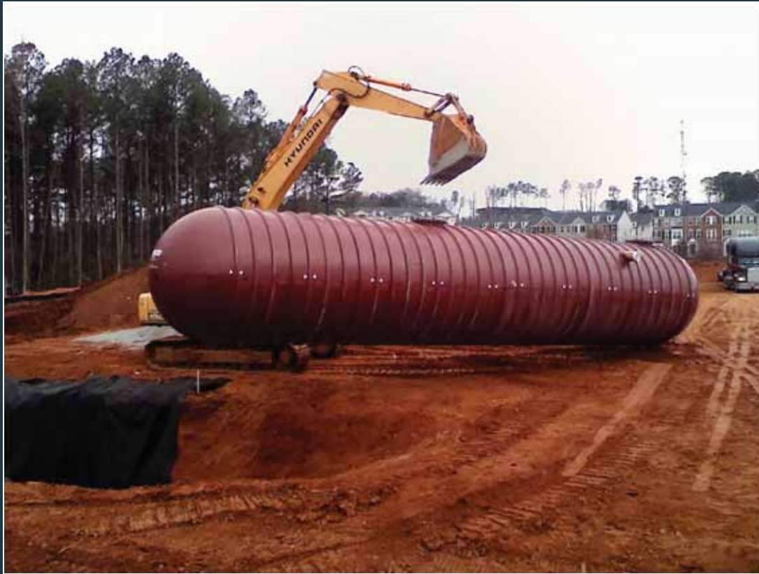
33,000 GALLON TANK - ADVANCED ALPHARETTA GA
